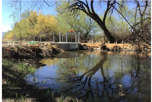
Coleman Creek – Olmstead Park Project- The point of diversion was moved upstream where a new headgate was installed with a fish screen. After removal of structure and installation of pedestrian bridge for access between the sprinkler system and the new diversion and pump station.
