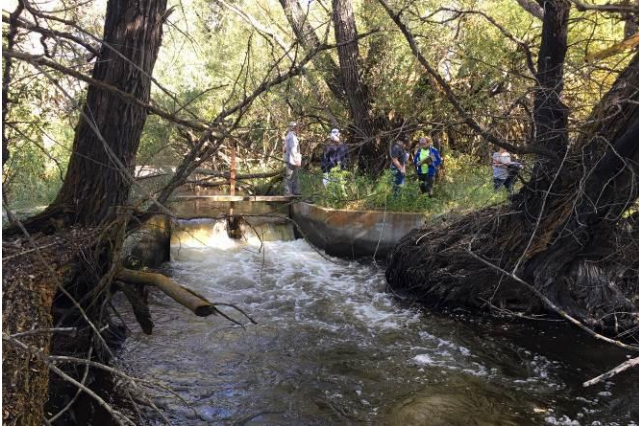
Coleman Creek – Olmstead Park Project- Concrete diversion structure was unscreened & a fish passage barrier.
